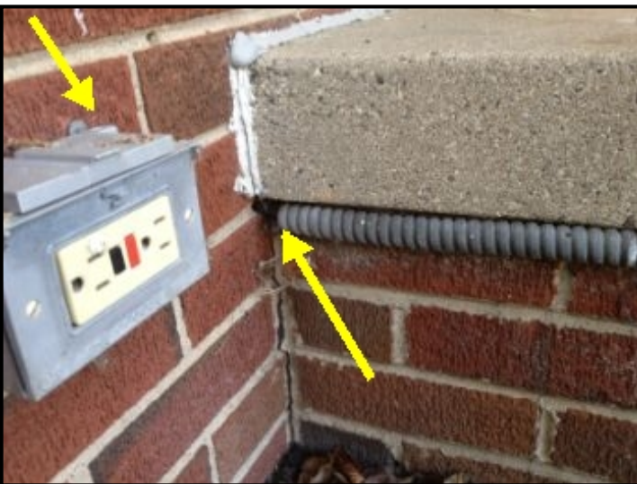
Broken GFI cover / exposed wires routed through brick wall
