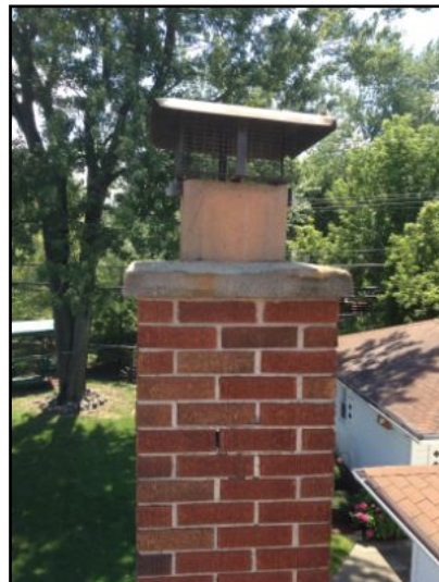
Roof Vent Caps
