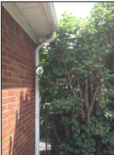
trim vegetation at least 1 foot from wall
