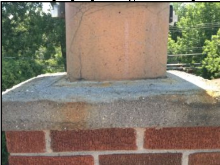
chimmney cap ok . monitor annually
