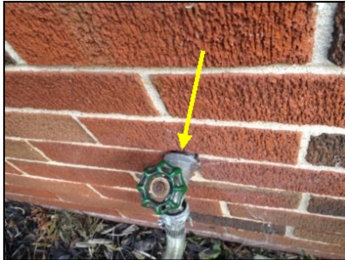
caulk needed at faucet to prevent water intrusion
