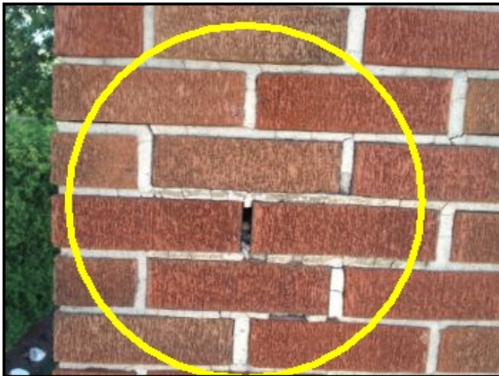
minor tuck pointing needed on chimney
