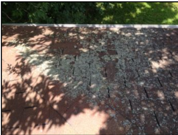
Garage roof beyond it's intended service life- OK at time of inspection
