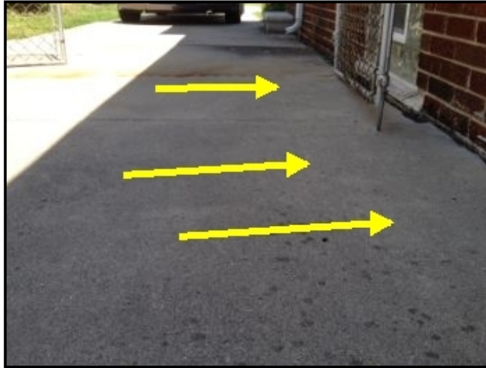
drive pitching wrong way toward house - possible water intrusion if left unrepaired
