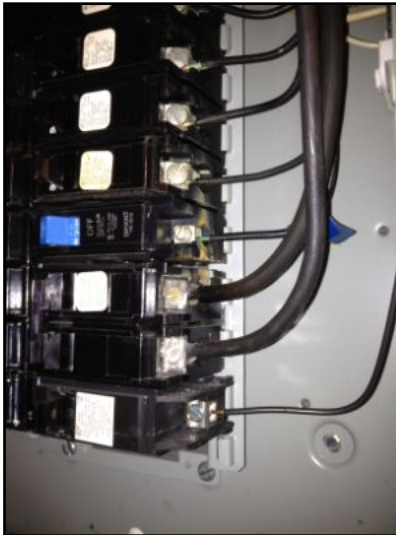
proper size aluminum service entrance cable
